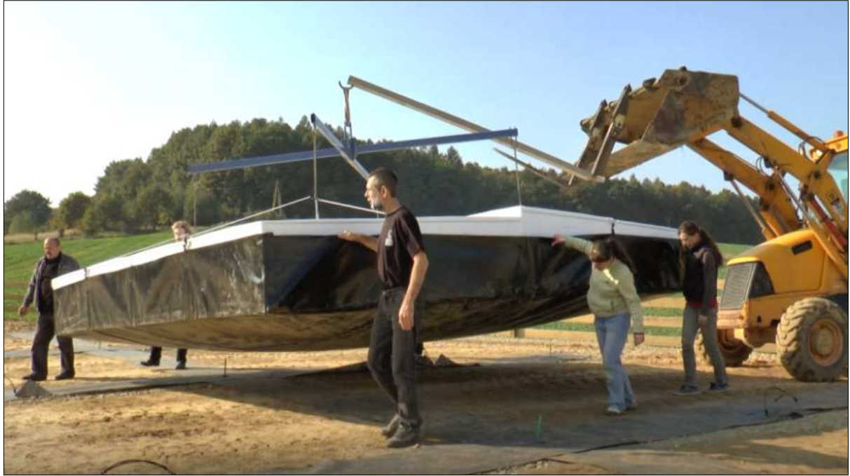
Figure 5: Installation of the high band antennas at the LOFAR station in Łazy near Kraków during September 2015 (courtesy: B. Śmieriak).
