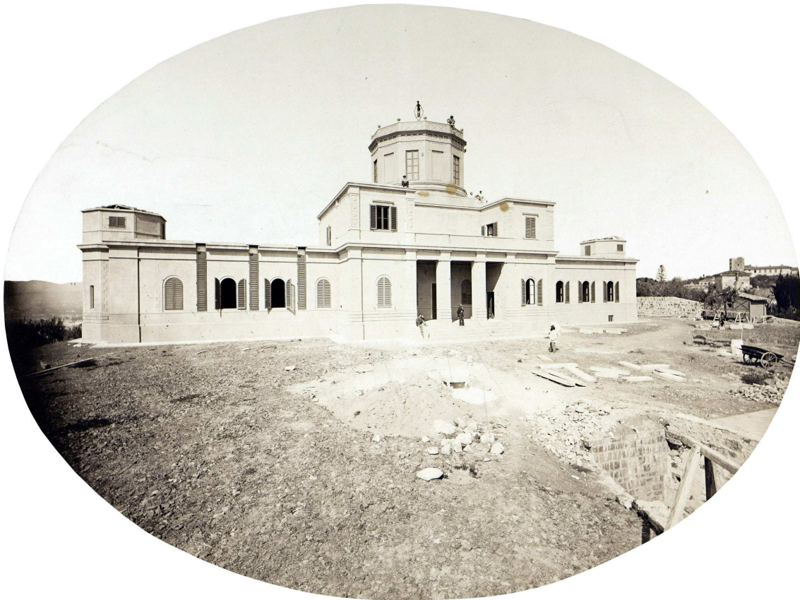
Figure 15: Finishing the construction of Arcetri Observatory, presumably in summer 1872 (courtesy: F.lli Alinari, Firenze. Museo Galileo, Firenze).
