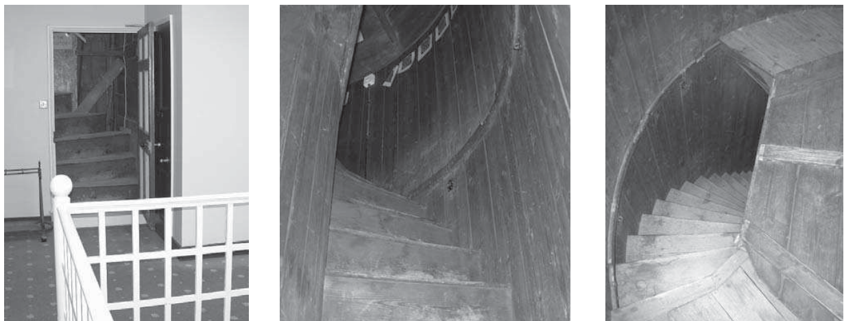
Figure 10. Left: The hidden staircase on the first floor Athenæum landing. Centre: The final curve of steps leading into the observatory dome. Right: The stairs viewed from inside the dome through the trap door.
